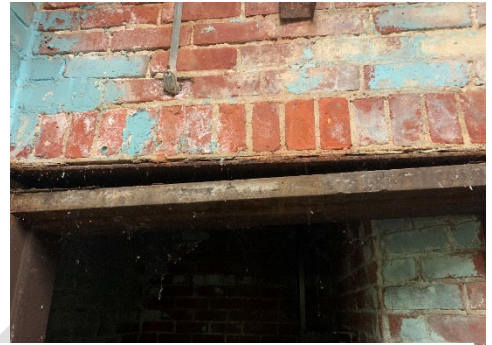
20: Door Opening Lintel in Boiler Room
