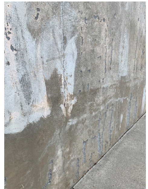
1222: Cracked Exterior Face of Existing Foundation Wall
