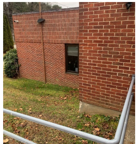
3: Partial Exterior Elevation - Spalled Corner of Concrete Foundation
